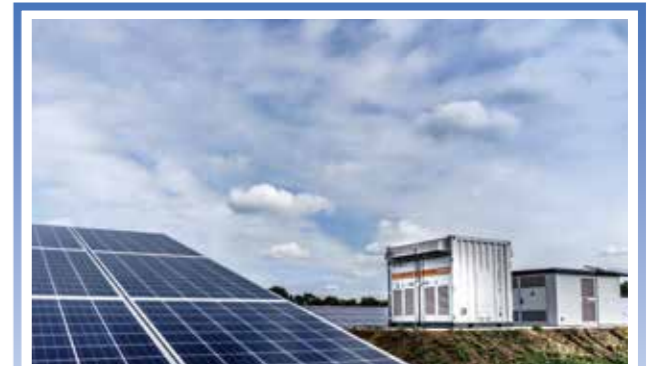
Energy Storage System 储能项目
